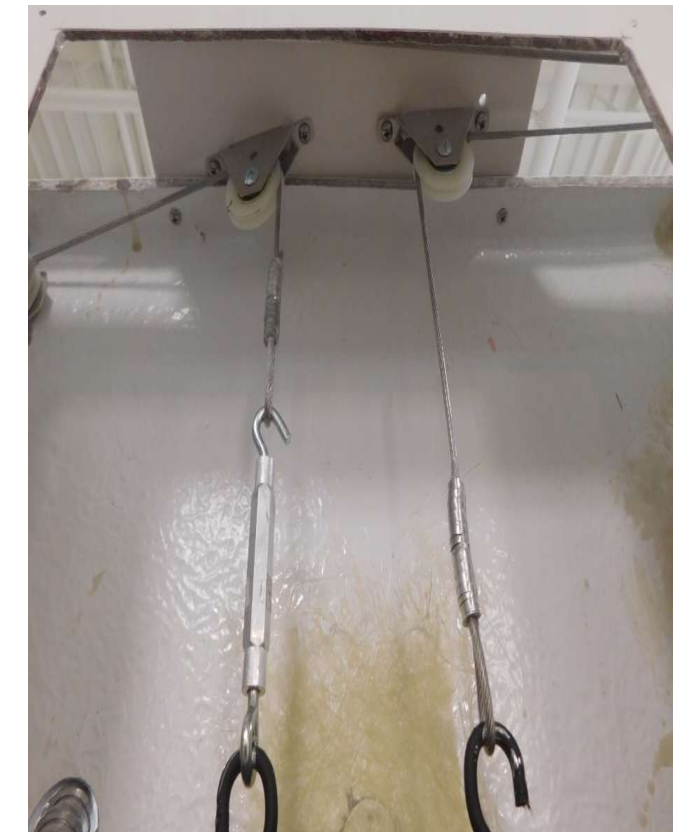
Note Location of cables inside of hood.
